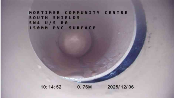
1, 00:00:07, 0.76 m Open joint, large
